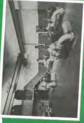
Water processing pumps
