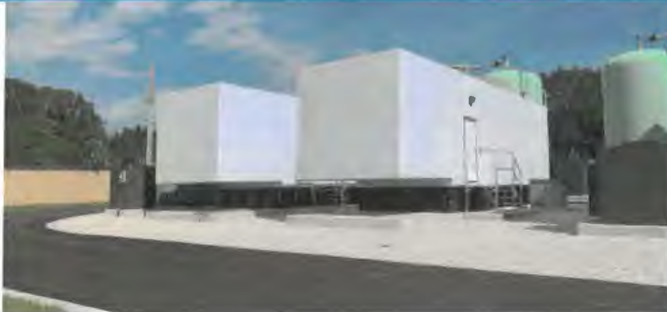
* Emergency Gen Sets Conway
