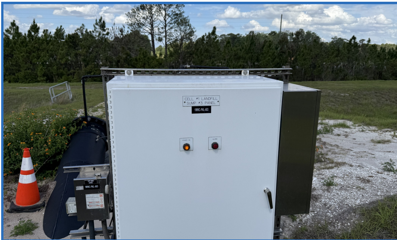
Outside of Control Panel Cabinet for Cell 1, Sump 3
