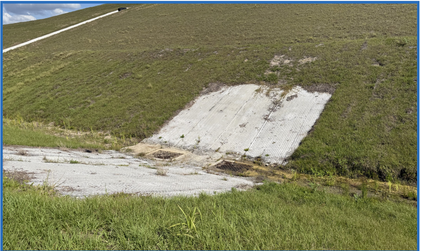
Fabriform with Inlets to Wet Detention Pond in Stormwater Ditch South of Cell 1
