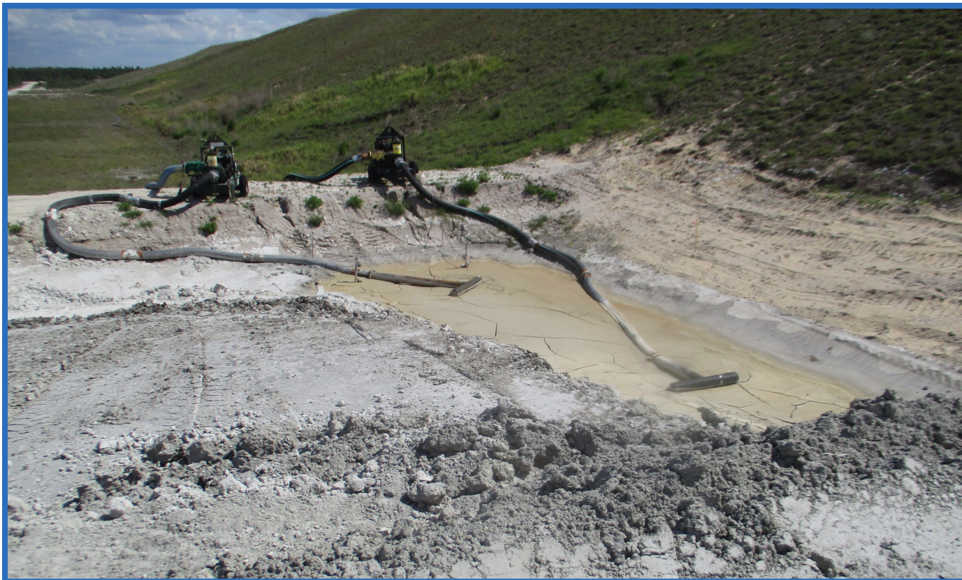
Diesel Auxiliary Pump with Intake Deployed in Cell 2
