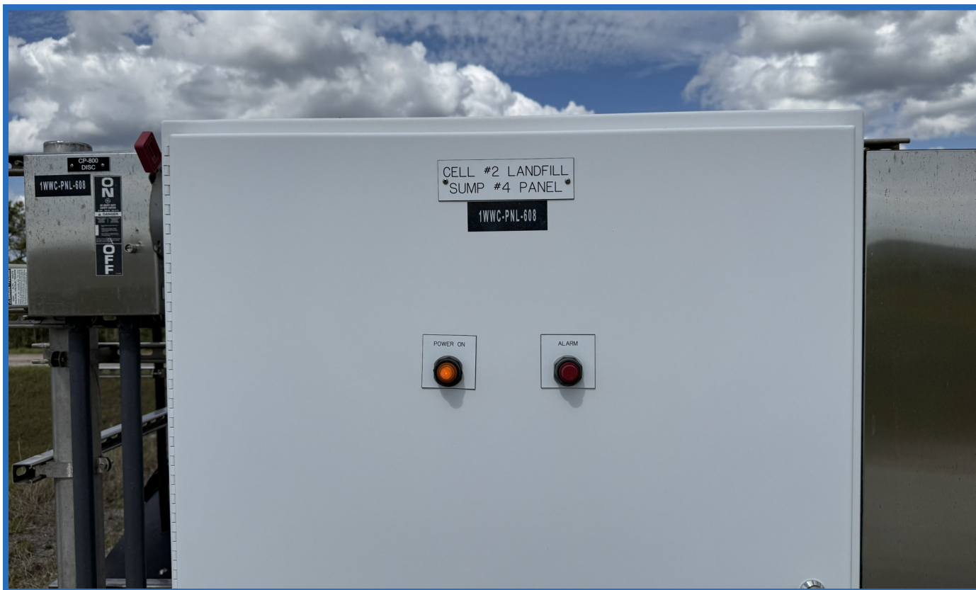
Outside of Control Panel Cabinet for Cell 2, Sump 4
