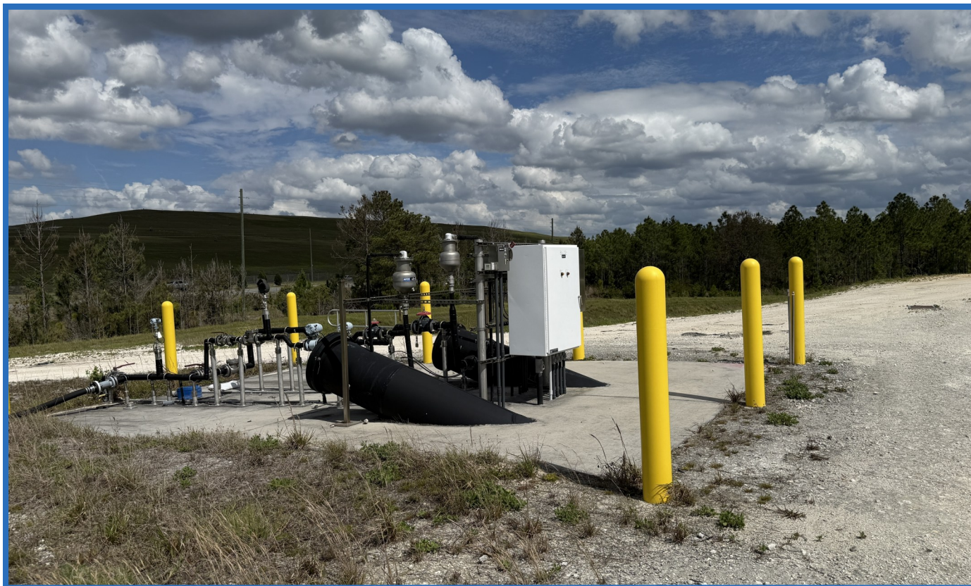
Leachate Pump Station for Cell 2, Sump #4
