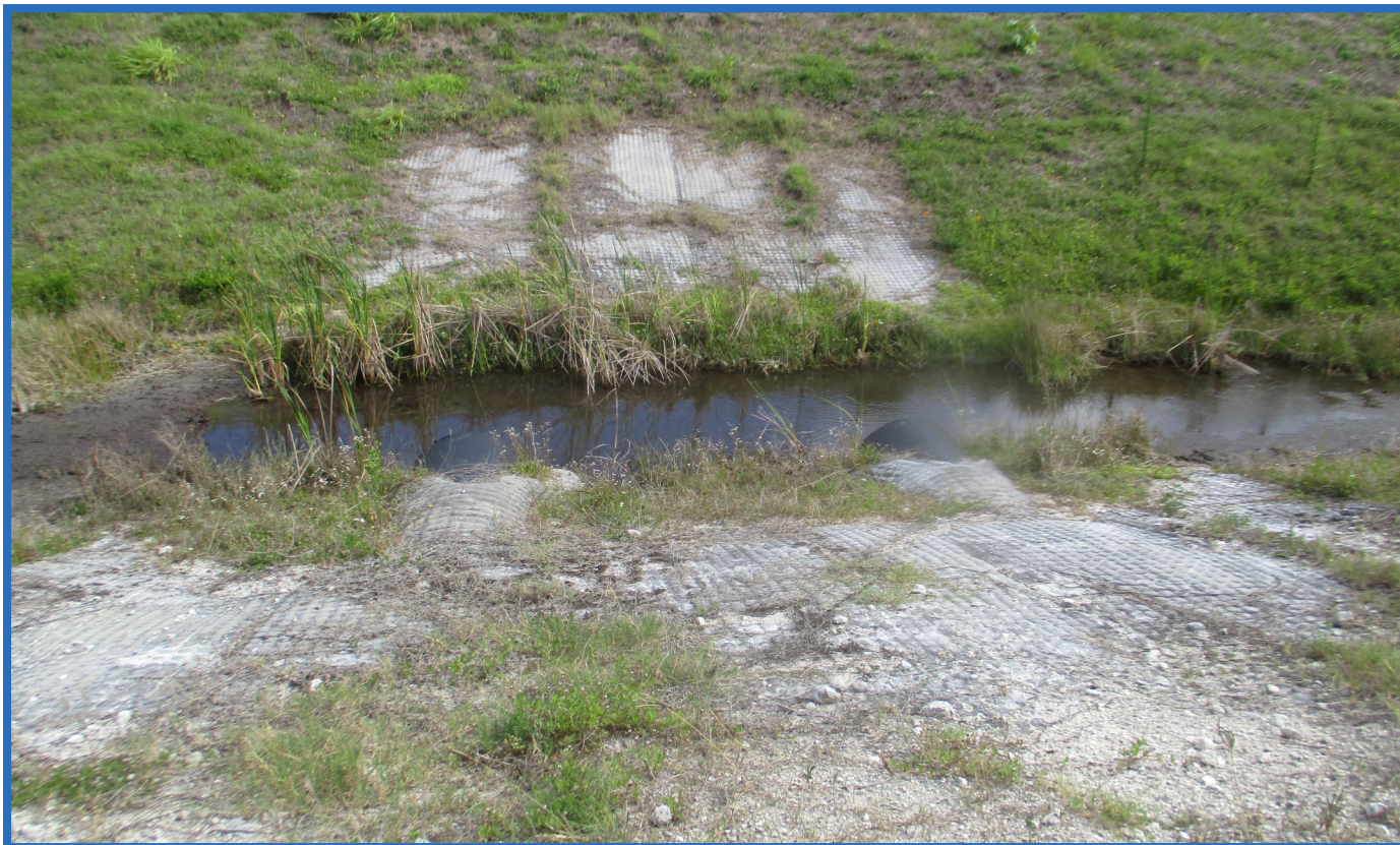
Fabriform with Discharge Pipes from Wet Detention Pond into Perimeter Stormwater Ditch (Looking Northwest from Perimeter Dike)
