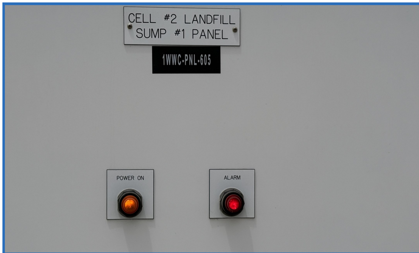
Outside of Control Panel Cabinet for Cell 2, Sump 1
