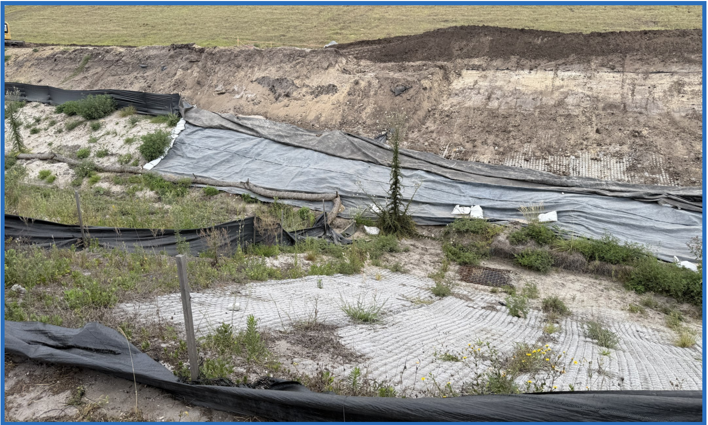
Fabriform with Inlets to Wet Detention Pond in Stormwater Ditch South of Cell 1 (Looking North from Cell 1 Perimeter Dike)
