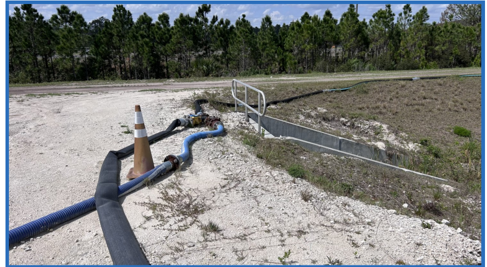
Connection of Discharge Pipelines from Auxiliary Pumps to Leachate Force Main
