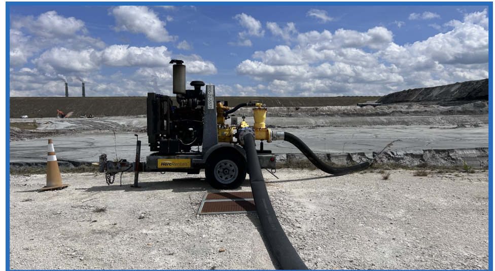
Diesel Auxiliary Pump with Intake Deployed in Cell 2, Subcell 1, Looking East
