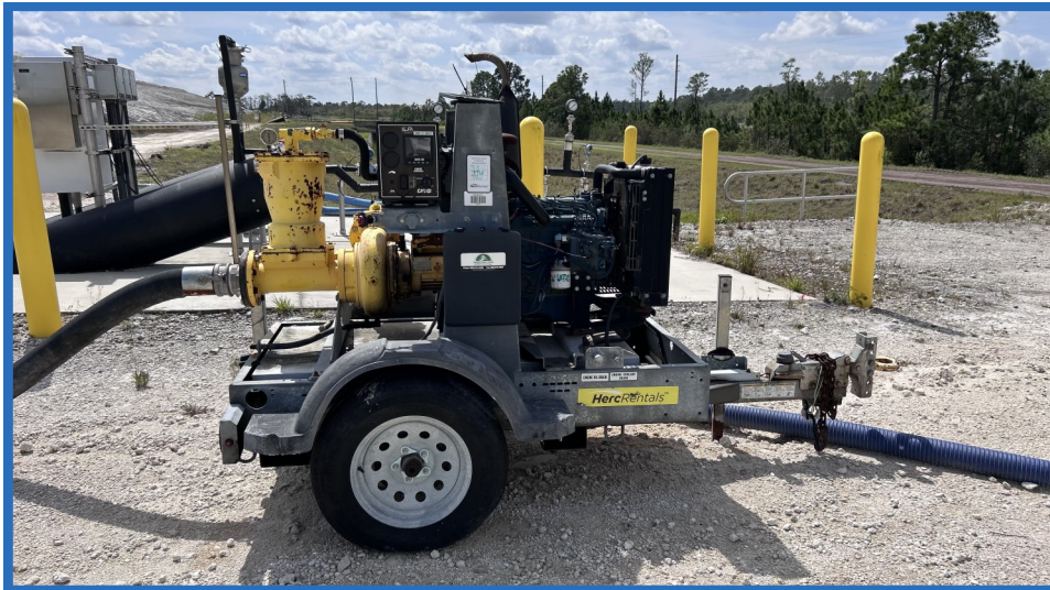
Diesel Auxiliary Pump with Connection to Leachate Force Main, Looking South
