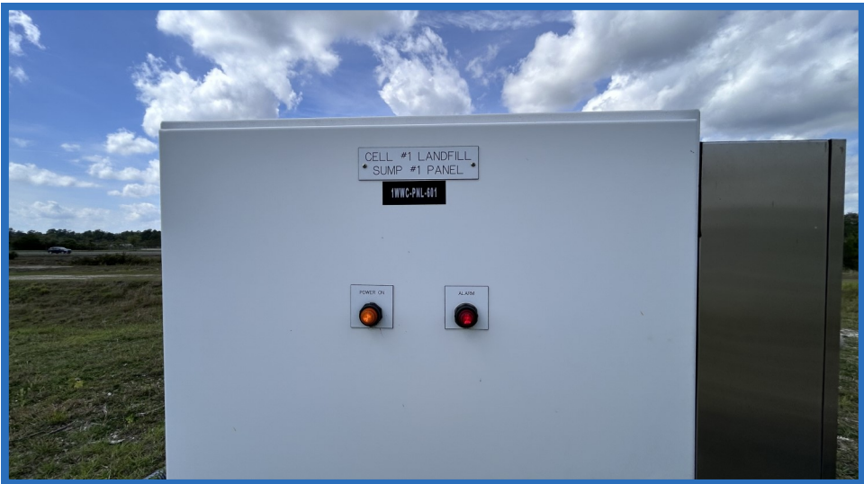
Outside of Control Panel Cabinet for Cell 1, Sump #1
