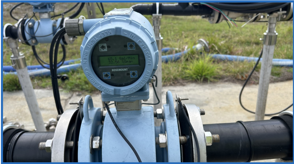
Leachate Flow Meter for Cell 1, Sump #1
