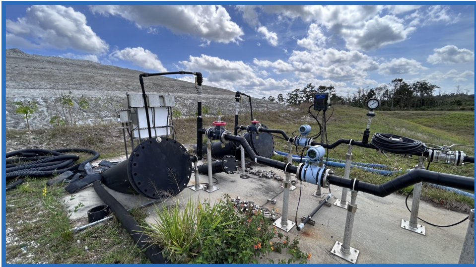
Leachate Pump Station for Cell 1, Sump #1
