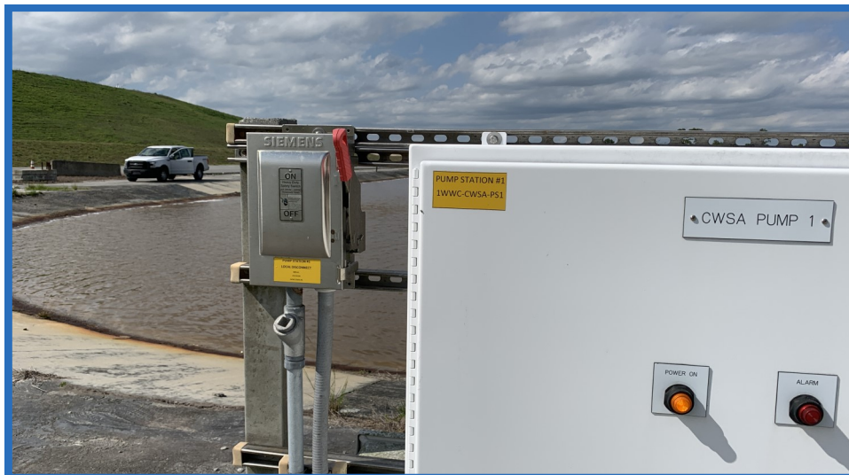
Outside of Control Panel Cabinet for CWSA Runoff Pond Pump 1
