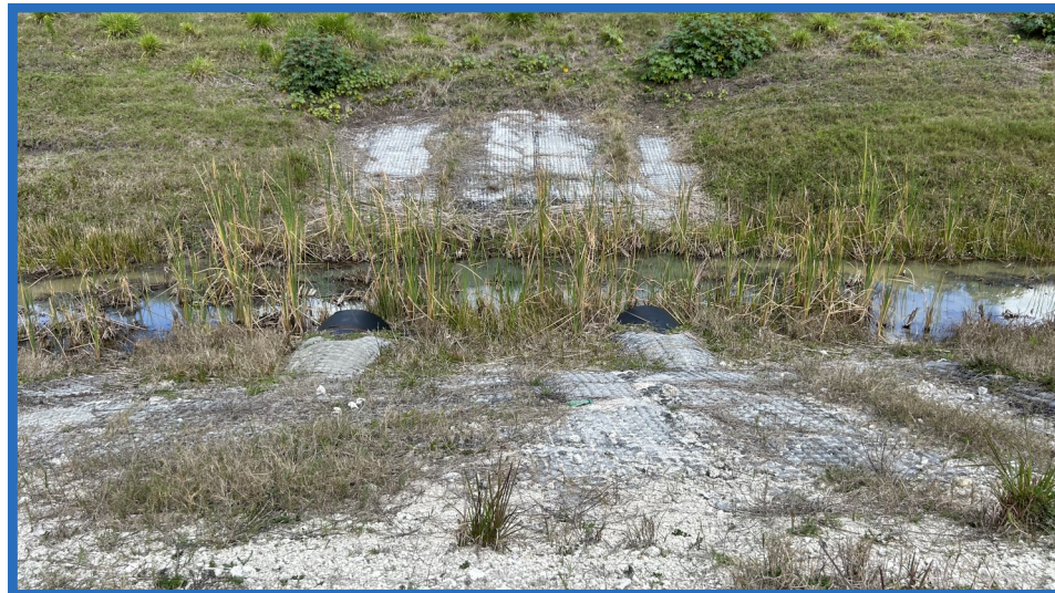
Fabriform with Discharge Pipes from Wet Detention Pond into Perimeter Stormwater Ditch, Looking North-Northwest from Perimeter Dike/Road
