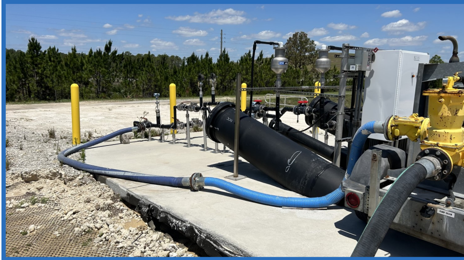
Connection of Discharge Pipeline from Auxiliary Pump to Leachate Force Main via Pump Station
