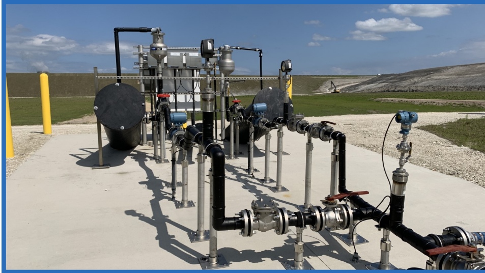
Leachate Pump Station for Cell 2, Looking East
