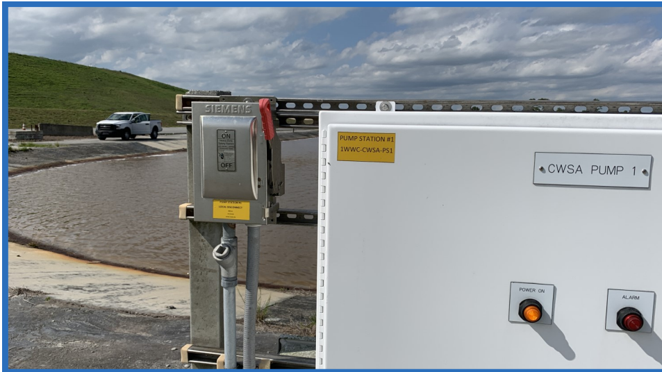
Control Panel for CWSA Runoff Pond Pump 1
