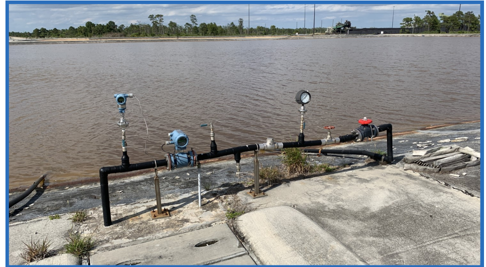
Meters, Gauges, Valves, and Cleanout Sump for CWSA Runoff Pond Pump
