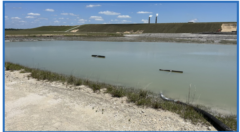
Intakes for Auxiliary Pumps in Preceding Photograph Deployed in Cell 2
