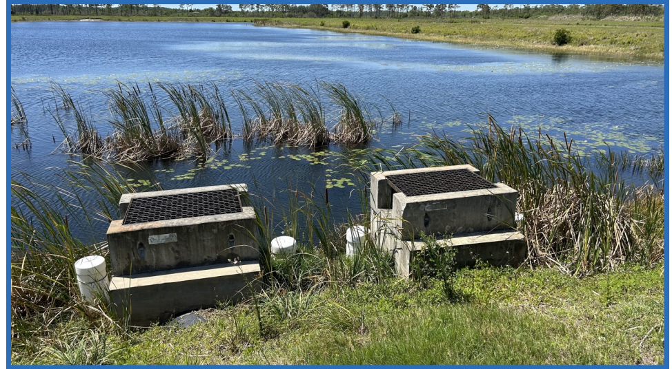
Discharge Structures for Wet Detention Pond, Looking South-Southwest
