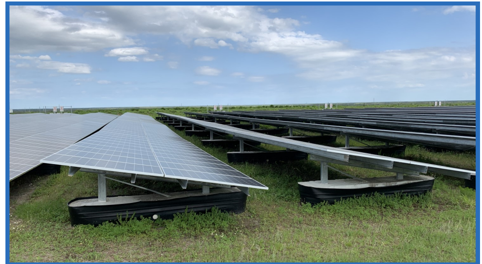
Photovoltaic Solar Panels on Top of Closed Vertical Expansion of Original CWSA, Looking Southeast
