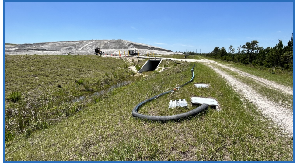
Connection of Discharge Pipeline from Auxiliary Pump Directly to Leachate Force Main
