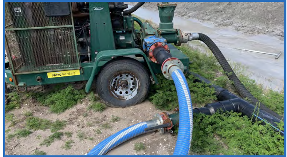
Closeup of Auxiliary Pump in Preceding Photograph Showing Connection to Discharge Pipeline
