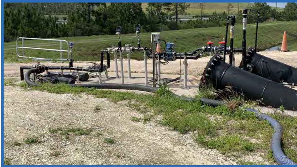
Closeup of Piping Connection in Preceding Photograph
