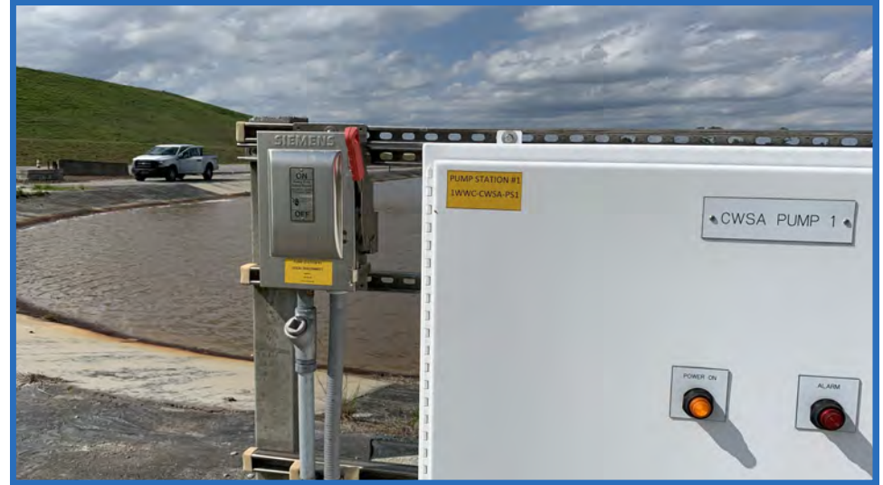
Control Panel for CWSA Runoff Pond Pump 1
