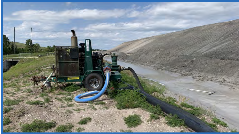
Diesel Auxiliary Pump with Intake Deployed in Cell 1 and Discharge Pipeline
