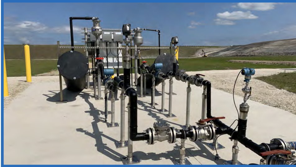
Leachate Pump Station for Cell 2, Looking East
