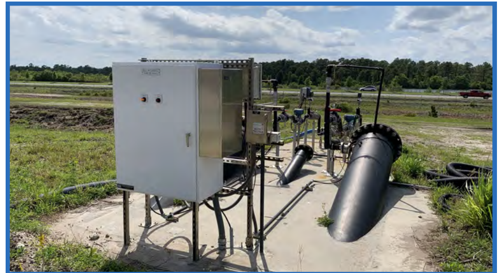
Leachate Pump Station in Sump #1 on the West Side of Cell 1, Looking West
