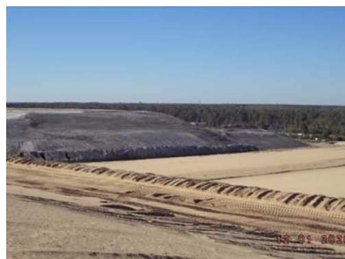
Cell 1 - disposal area
