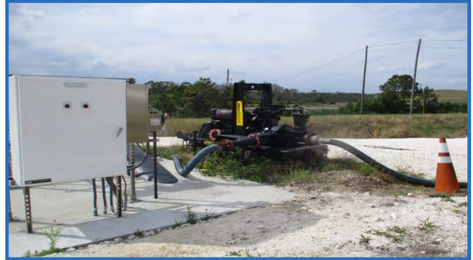
Auxiliary Pump Deployed at Sump 2 to Pump Station Discharge Piping
