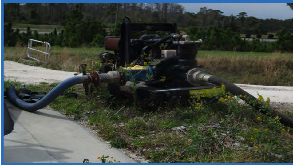
Auxiliary Pump Deployed at Sump 3
