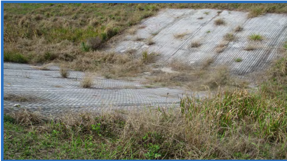
Fabriform with Inlets Connected to Pipes Discharging to Wet Detention Pond, Looking Northwest
