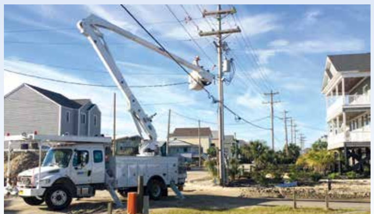
OUC line techs got straight to work after arriving in Conway, SC to help Santee Cooper restore customers out of power following Hurricane Matthew.
