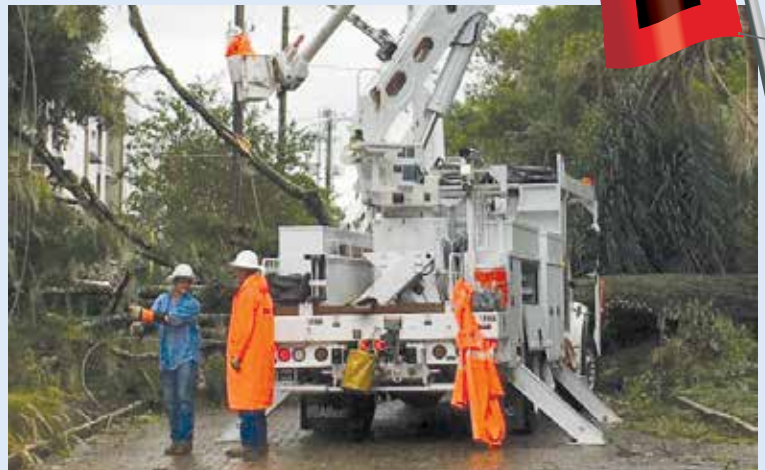
OUC line techs work between fallen tree limbs to restore power in downtown Orlando after the storm.
