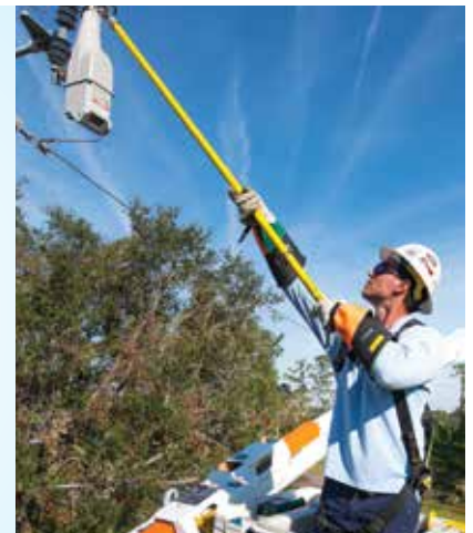
Roger McBride, Line Technician, installs a TripSaver II device on a test line at the Pershing Operations Center.
