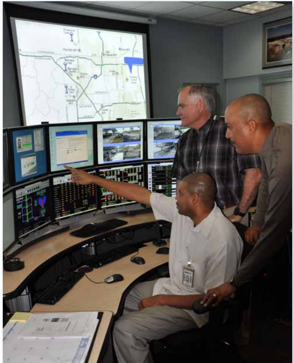
Water Production control room
