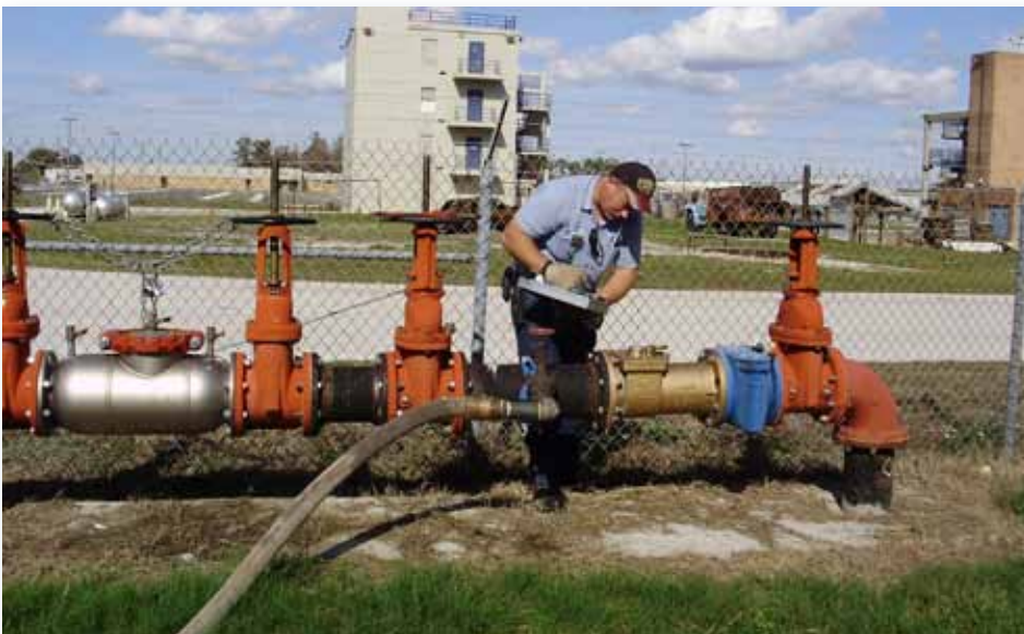
Lynn Benson, Distribution Technician
