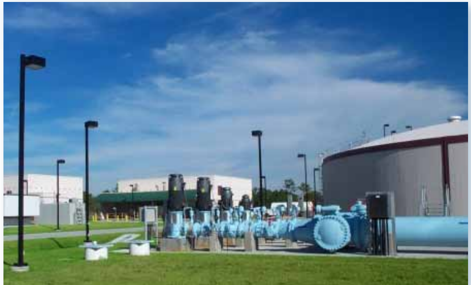
Stanton Water Facility
