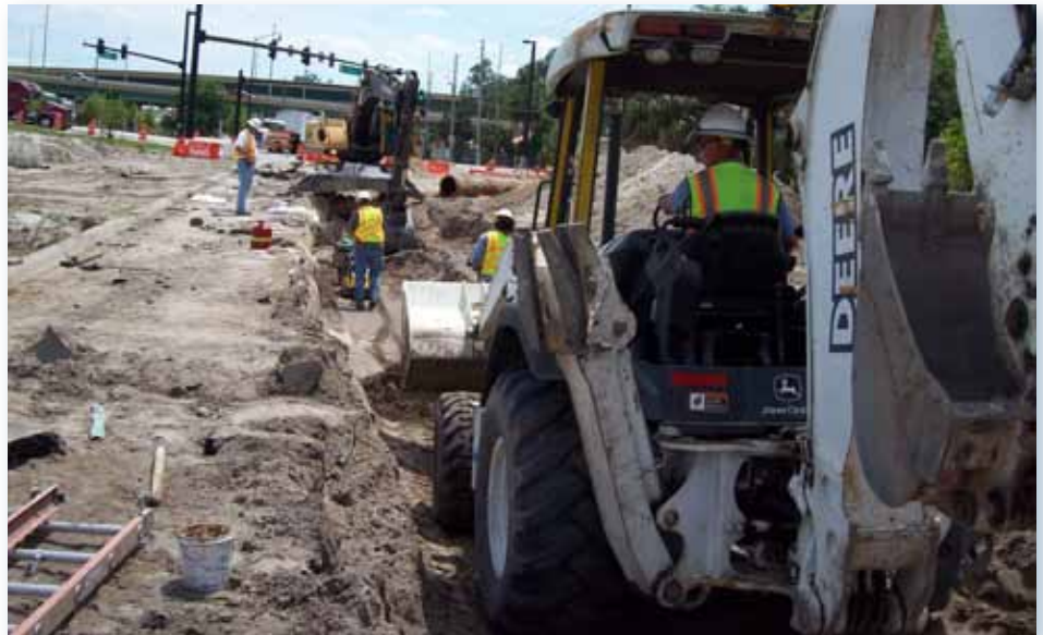
Water Distribution Crew rely on the GIS system maps to maintain and construct water pipes on Anderson Street and Division Avenue
