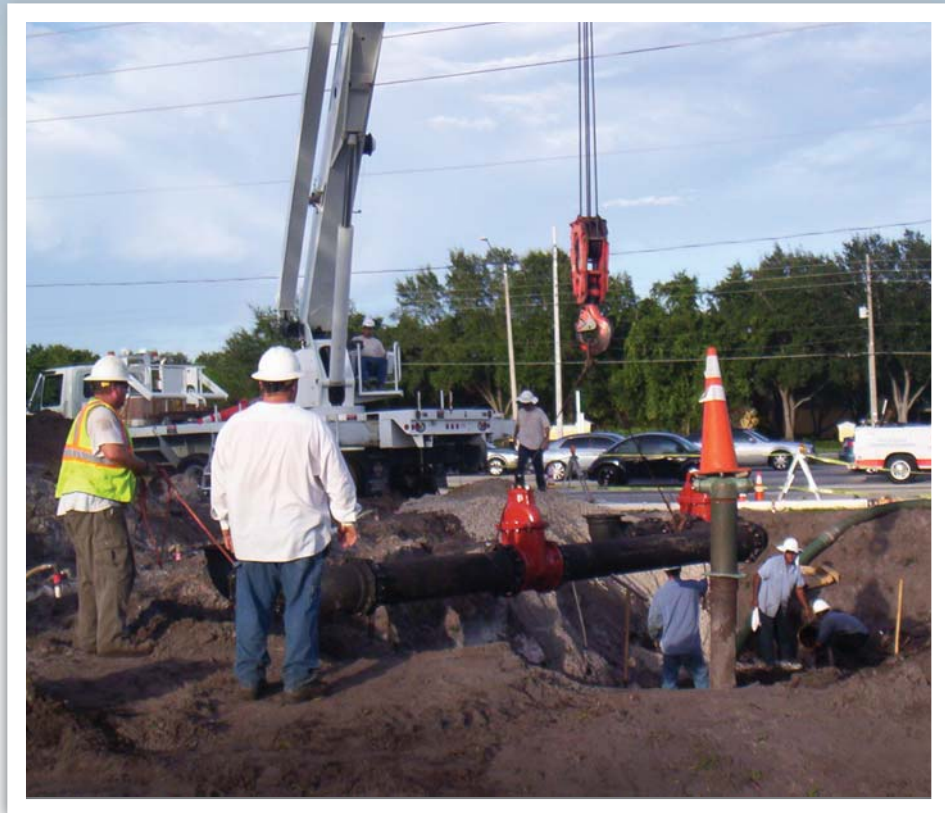
10-inch water meter at Valencia College on Kirkman Road
