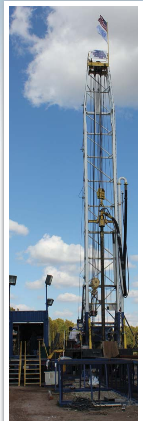
Drilling of a multi-zone deep monitoring well in OUC's Southeast Water Resource Area
