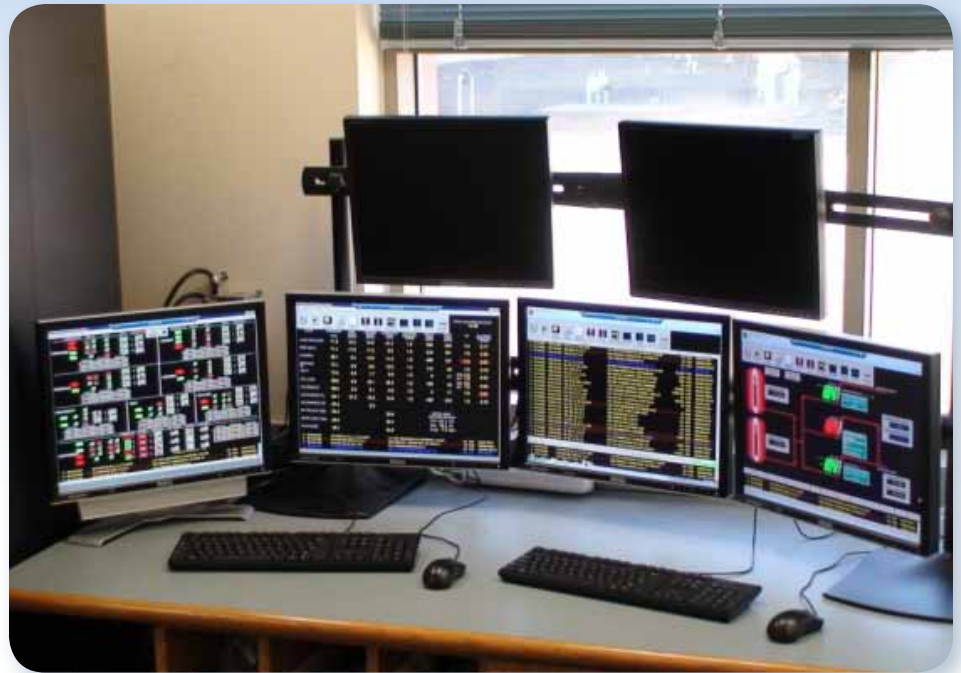
Operator Station at the Southwest Water Treatment Plant
