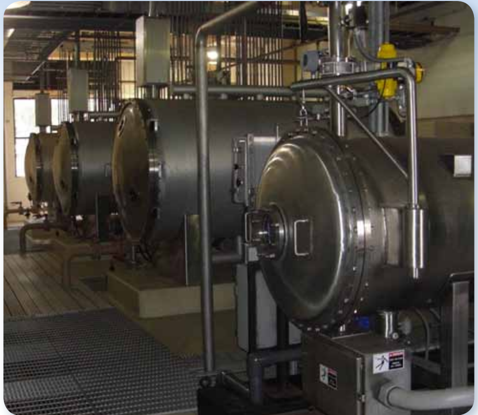
Conway WTP-ITT Wedeco (foreground) and PTOC (rear) Ozone Generators
