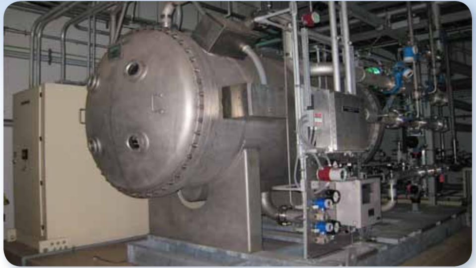
Sky Lake WTP - Day Ozone Generator Manufactured by Ozonia
