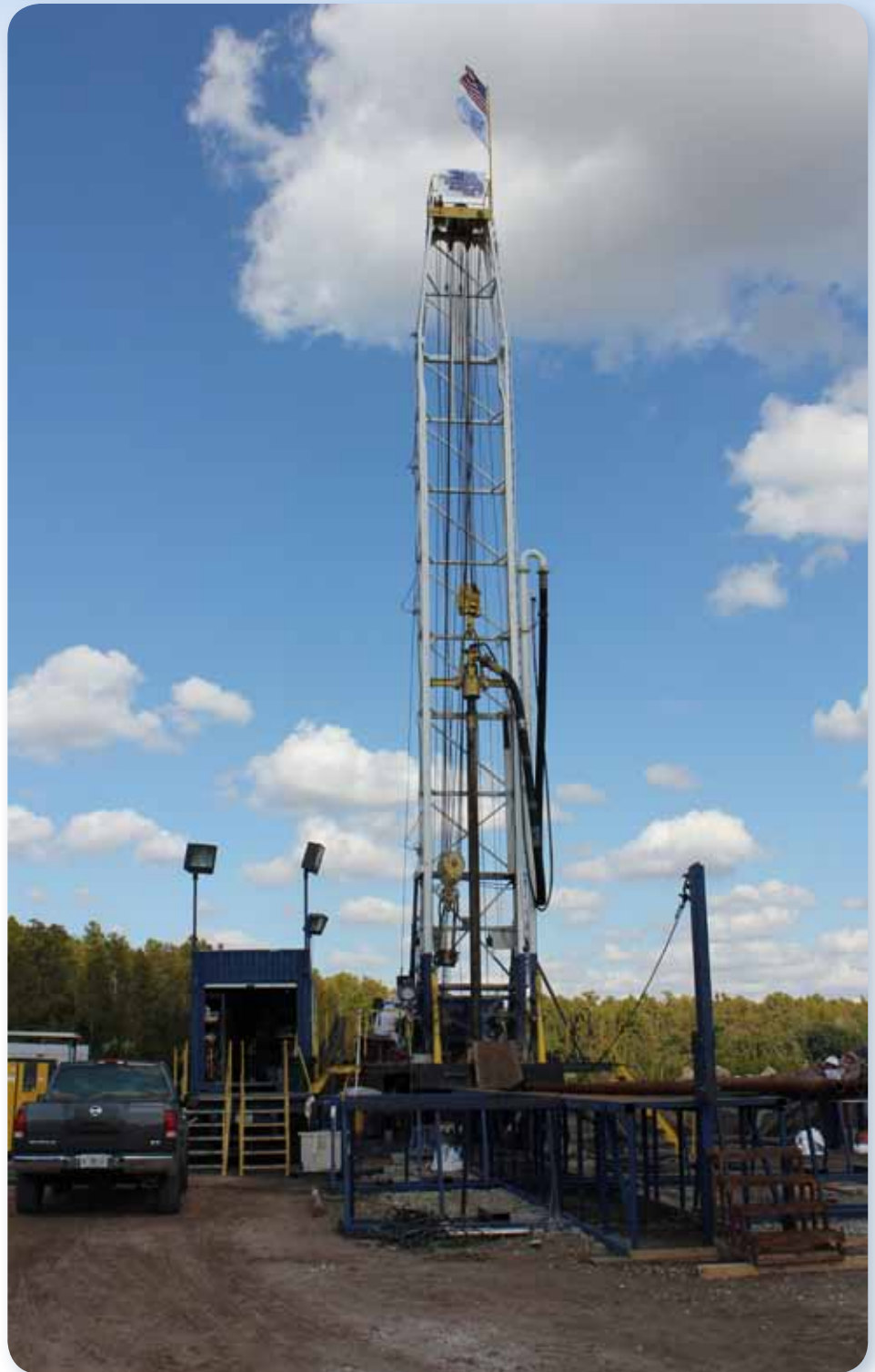
Drilling of a multi-zone deep monitoring well in OUC's Southeast Water Resource area
