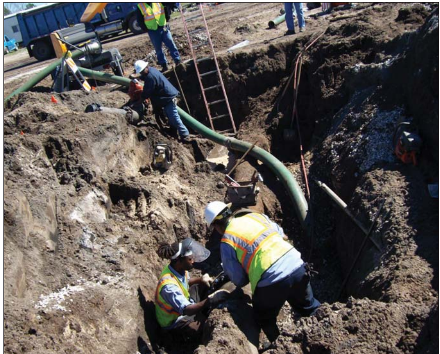
Water Distribution crews rely on accurate maps prepared by the Technical Services Section to locate underground pipes.
